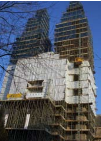
Over 36 miles of scaffolding was used in the 2004/5 restoration of the West Front.
