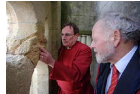
The Dean, Dr Christopher Hardwick, and Sir Barry Cunliffe (English Heritage) examine the damage to stonework on the central tower caused by wind, rain and salt-laden air.
